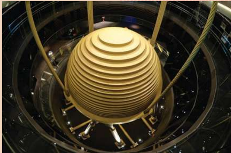
Photo 2. Close up view of TMD in Taipei 101 Tower.
