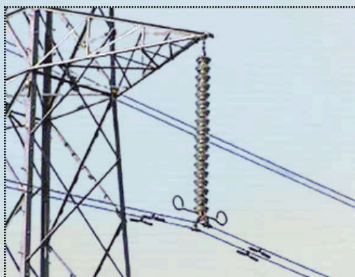
Photo 1. Dampers used to prevent aeolian vibration.
